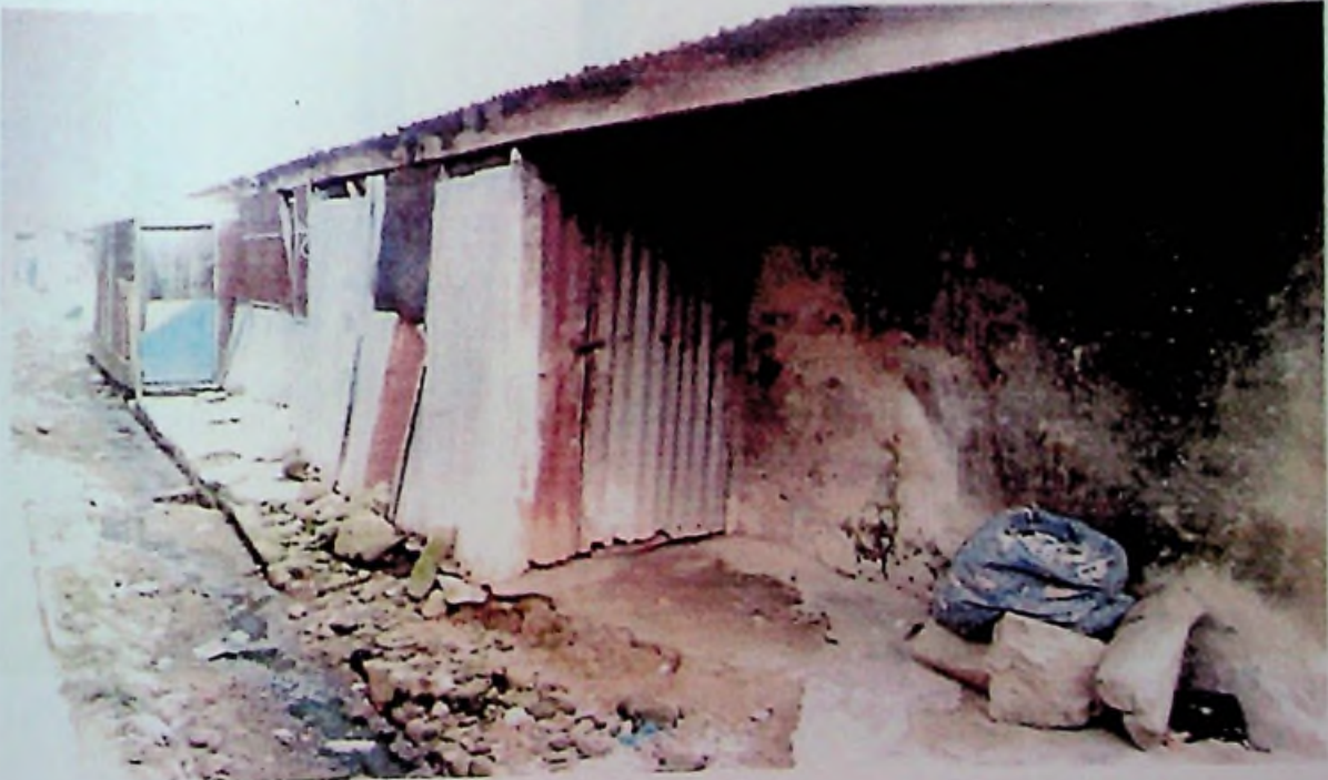
Plate 4.1: A Typical Poor Housing Condition
