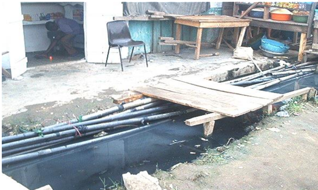
Plate 4.2: Water Pipe Line inside Drainage Channel.
